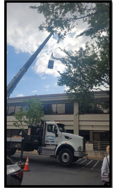
HVAC Replacement Following a Catastrophic Unit Failure
