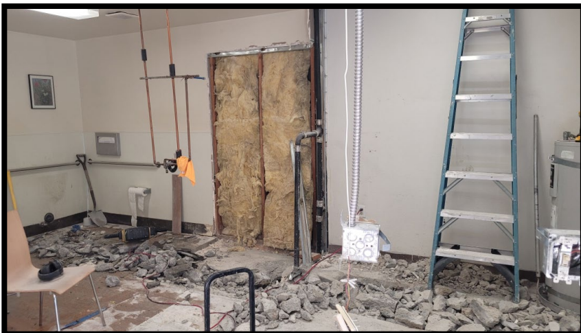
Pictured here, sewer pipe replacement and connecting to the adjoining suite began in the last quarter of 2025.
